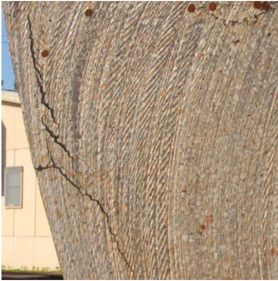
(A) Severe Sub-Parallel Cracking
