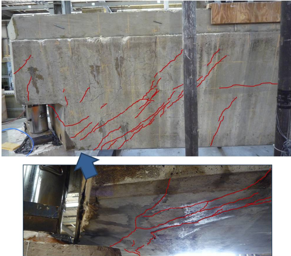
Figure 4-6: Post-Failure Cracking in Segment N-II
