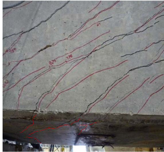
(B) Bottom-Side Anchorage Cracks
