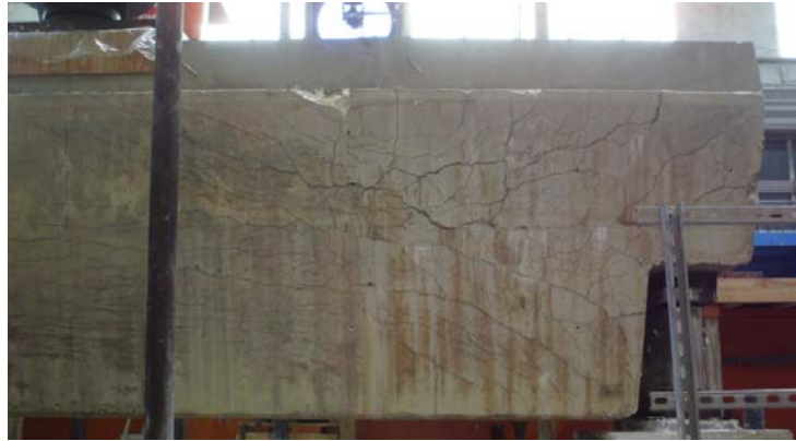
Figure 2-15: Premature Concrete Deterioration
