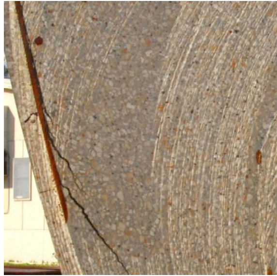
(B) Debonding of Transverse Reinforcement
