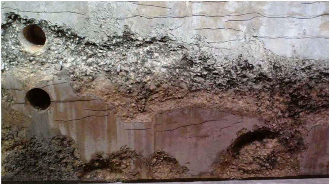
Figure 3-8: Example of Poor Consolidation
