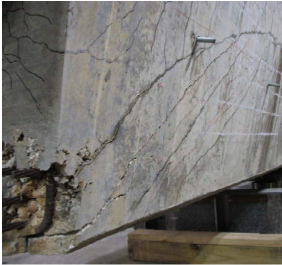
(A) Diagonal Cracking within Transfer Length
